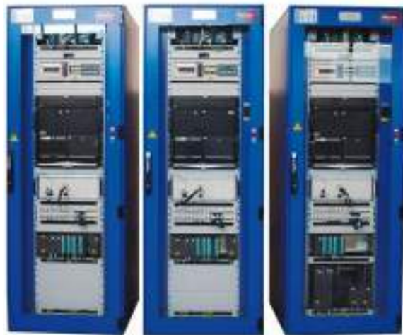
I&C Cabinets Procon Systems for ITER
