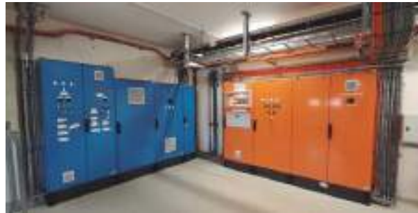
Electric cubicles - CERN AD TARGET
