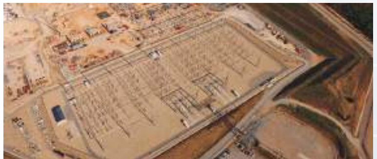
The very high voltage electrical substation on the south side of the platform (Photo IO EJJF Richie)
