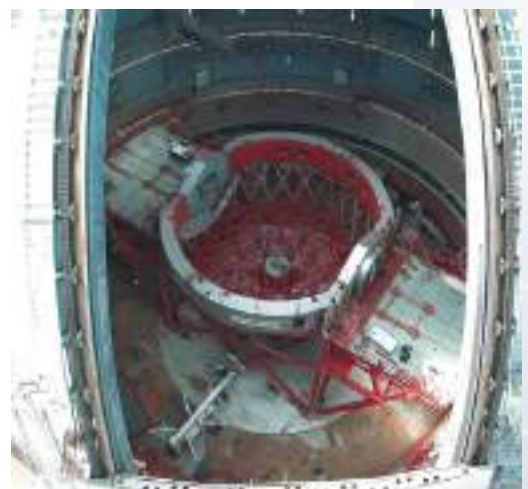
GranTeCan installation in La Palma
