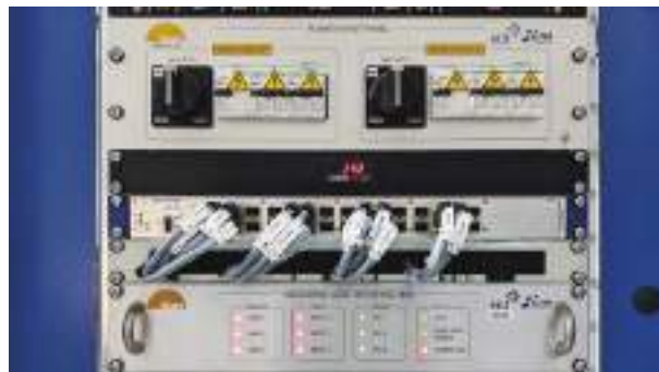
Power Input Panel and Discharge Loop Interface Box
