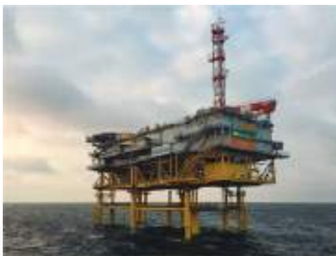
Iberdrola substation installed at german Wikingen offshore wind farm. Photo Iberdrola
