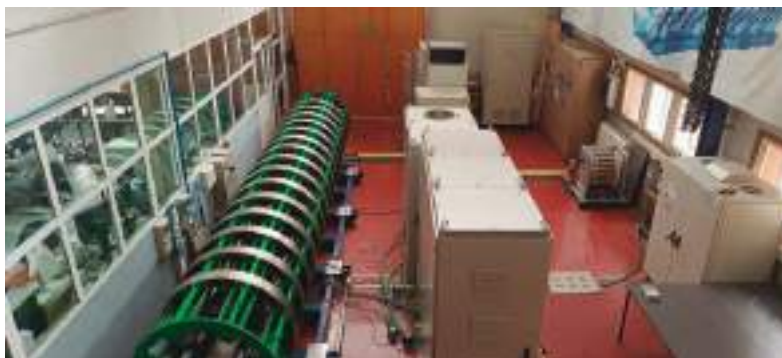
Facility for Testing Linear Generators for Wave Energy Conversion
