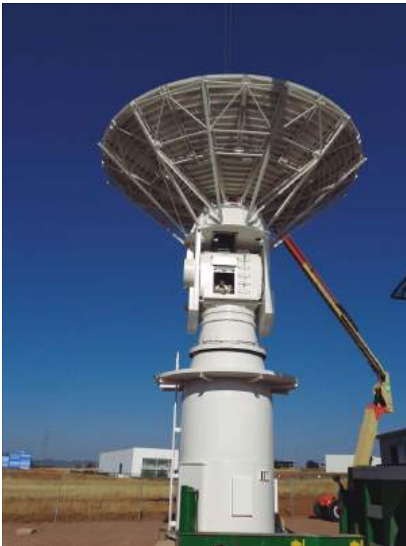
Deimos Ground Station - Elecnor Deimos - Integration of the 10 m TTC Ground Station for Deimos-2 Satellite, 2013
