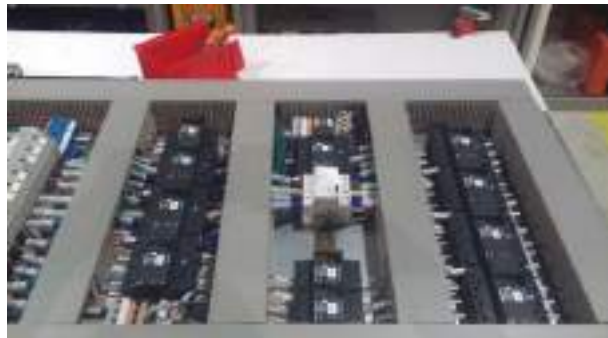
Lower part of the HSB01 distribution board
