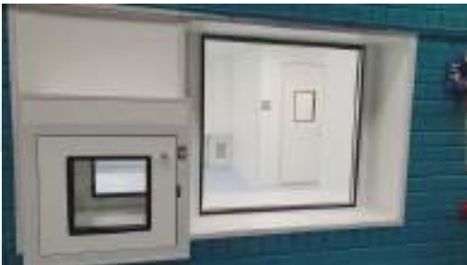
ARQUIMEA facilities - clean room
