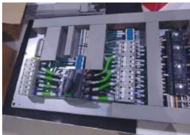
Upper part of the HSB01 distribution board including high current distribution devices
