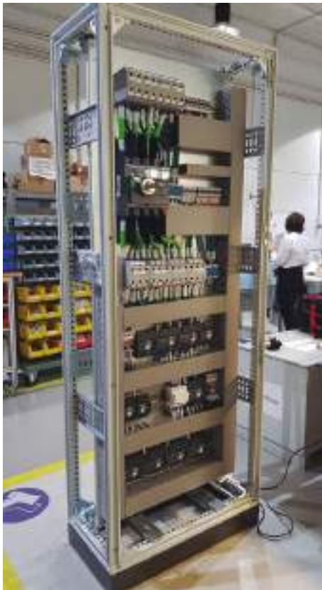
HSB01 distribution board
