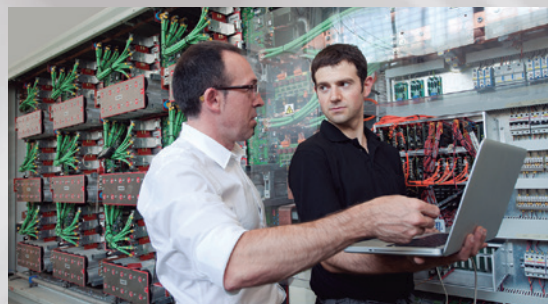
JEMA facilities ESS-Bilbao Project
