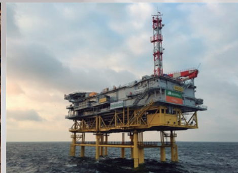
Iberdrola's substation installed at German Wiking offshore wind farm (Photo Iberdrola)
