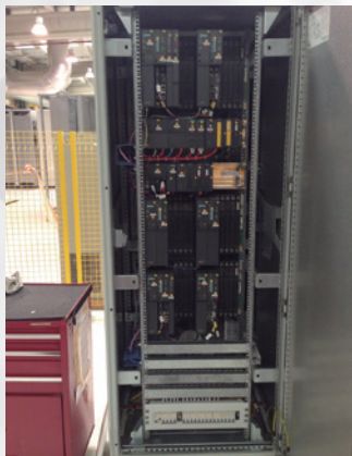
SCS-N Qualification Cubicle
