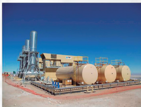
ALMA Multifuel Power Plant (2011)
