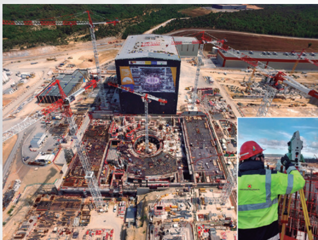
Aerial view of the central building (Tokamak Building) and the annex building (Assembly Hall) where the components of Tokamak are pre-assembled. (November 2016)
