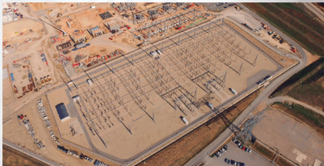
Electrifying- The very high voltage electrical substation on the south side of the platform (Photo ITER Organization/EJF Riche)
