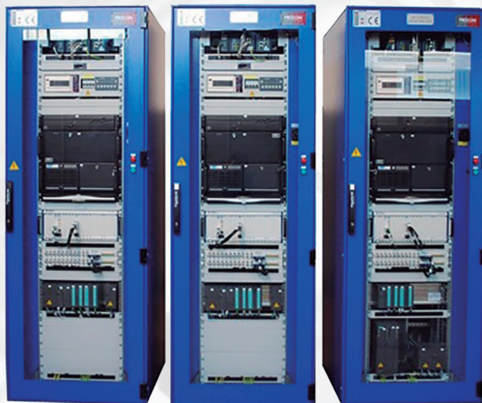
Procon I&C Cabinets Procon Systems For Iter
