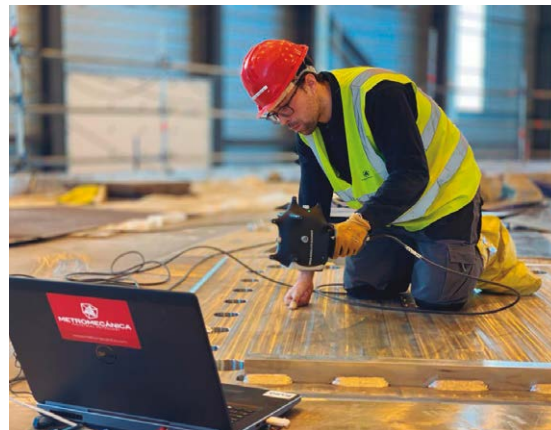
Measurement in ITER facilities
