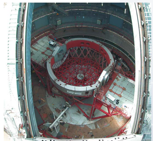
GranTeCan installation in La Palma
