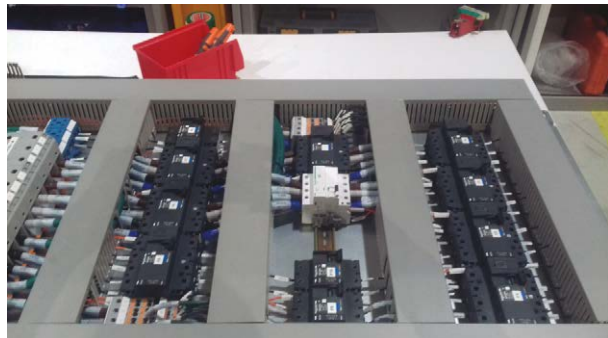
Lower part of the HSB01 distribution board
