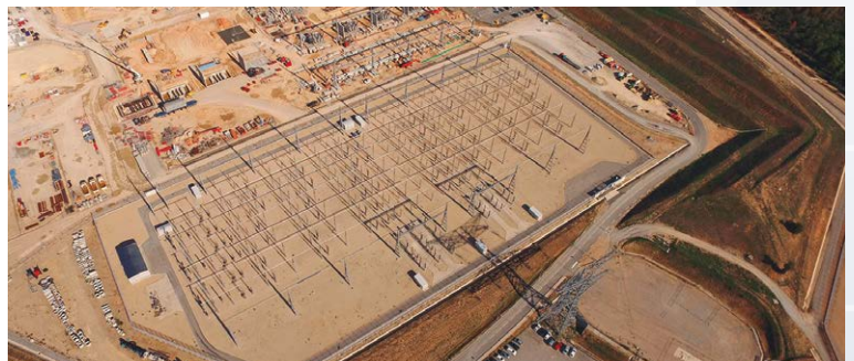
The very high voltage electrical substation on the south side of the platform (Photo IO EJP Richie)
