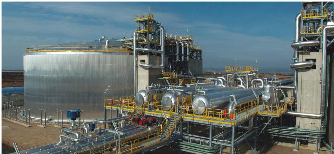
Thermal Energy Storage System in Thermosolar Power Plant
