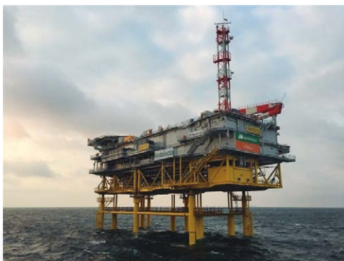
Iberdrola substation installed at german Wikingen offshore wind farm. Photo Iberdrola
