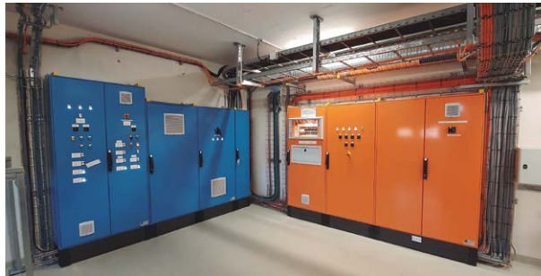
Electric cubicles - CERN AD TARGET
