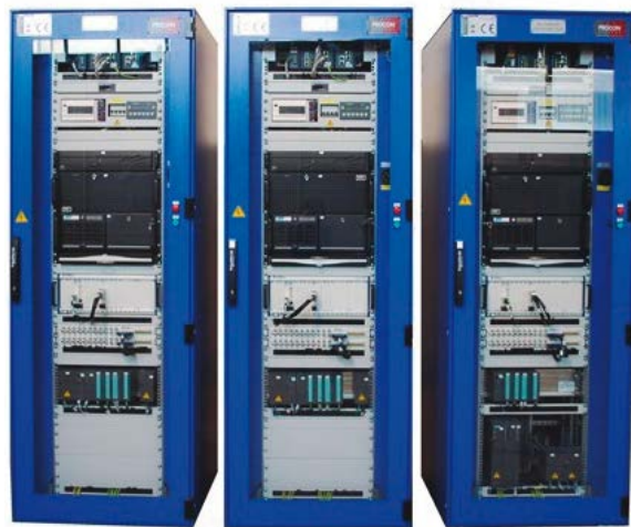
I&C Cabinets Procon Systems for ITER
