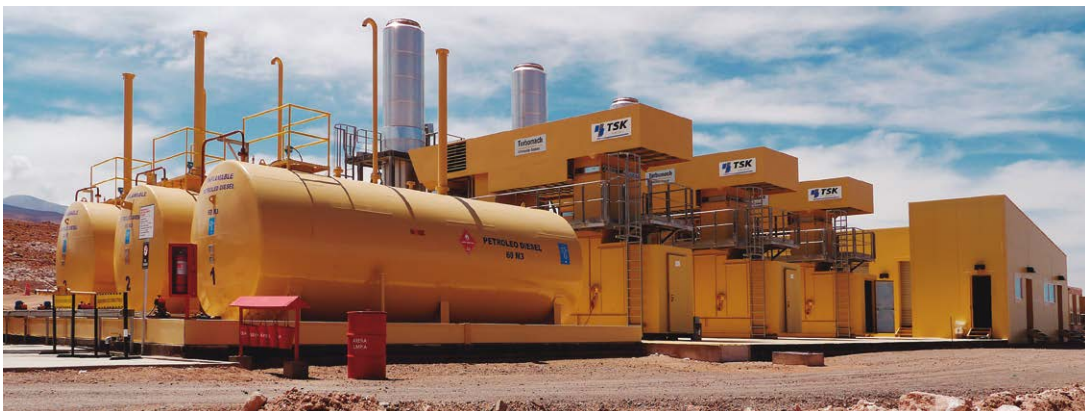
ALMA Multifuel Power Plant (2011)
