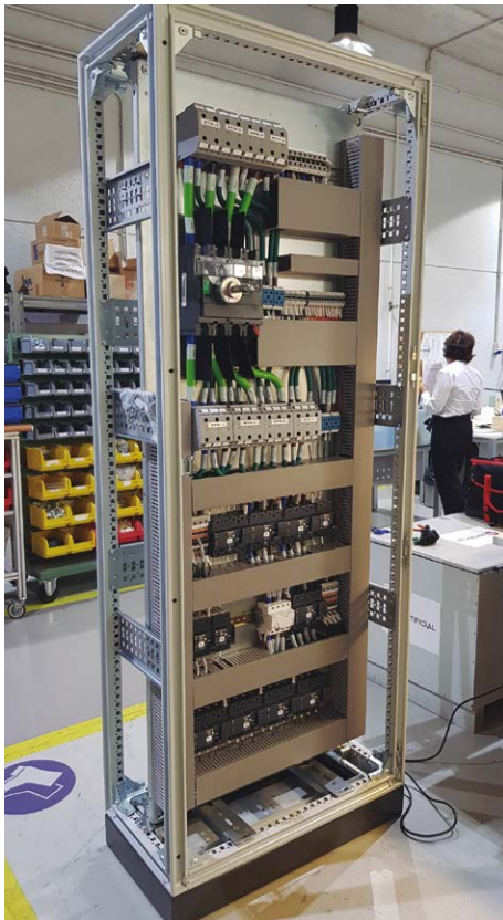
HSB01 distribution board
