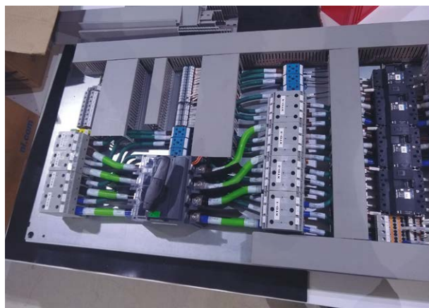
Upper part of the HSB01 distribution board including high current distribution devices
