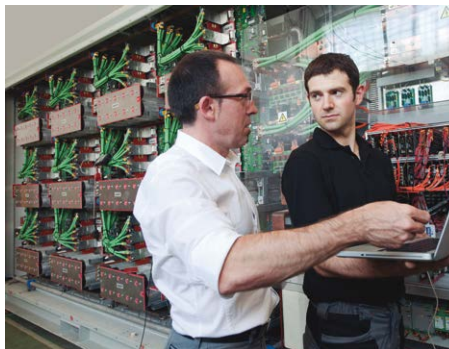
JEMA facilities ESS-Bilbao Project
