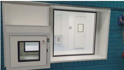
ARQUIMEA facilities - clean room
